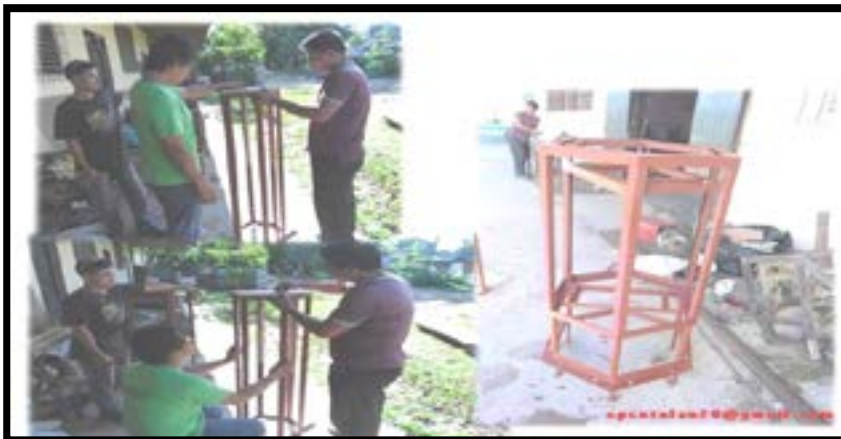
Figure 7. Inspecting the base structural frame of the charging station as shown in the picture.
