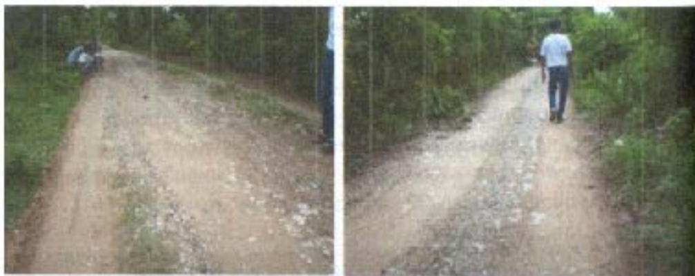
Picture of the remains of the original Road constructed by the American forces in Supang, Buenavista, Guimaras
