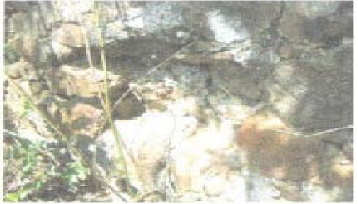
The hallow portion of the parapet facing the road where a slab of rock embedded on the wall marked "29 Inf. 1903", a mute autograph of the builders of the parapets but at present it is already gone.
